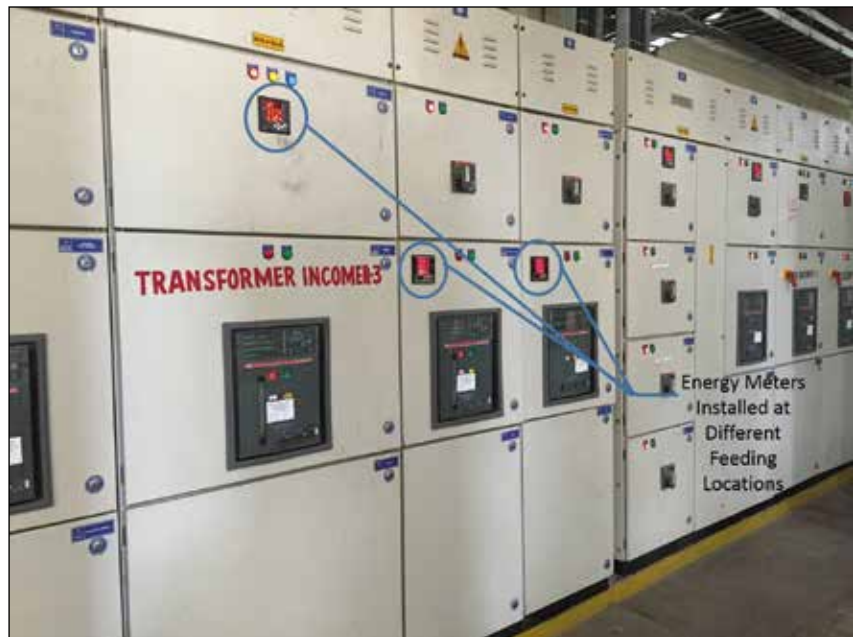
Figure 1: Installation of energy meters at different feeder locations easily executed at the panel level
